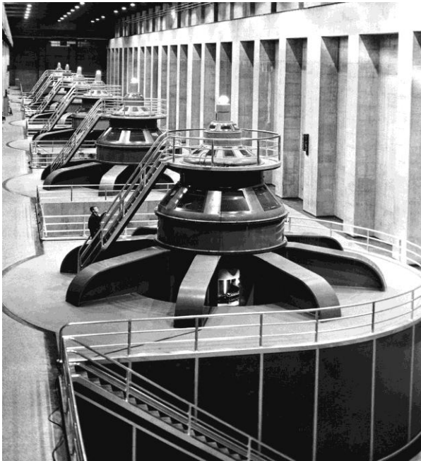
Fig.5 Six Turbines up close
