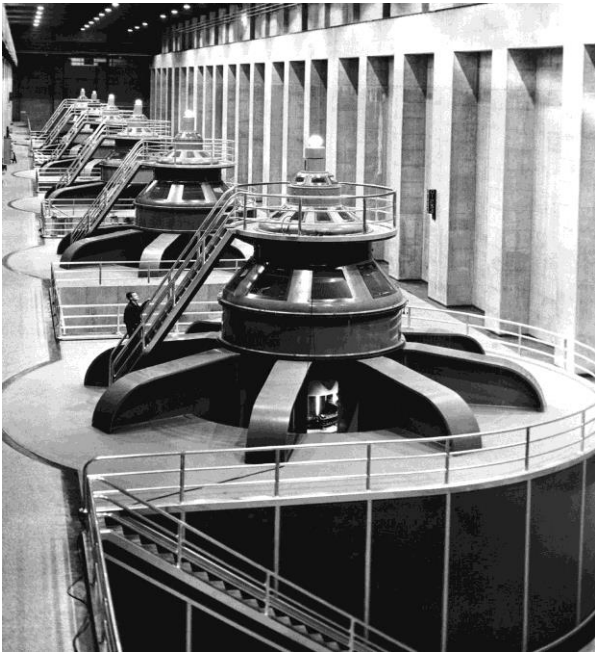
Fig.5 Six Turbines up close
