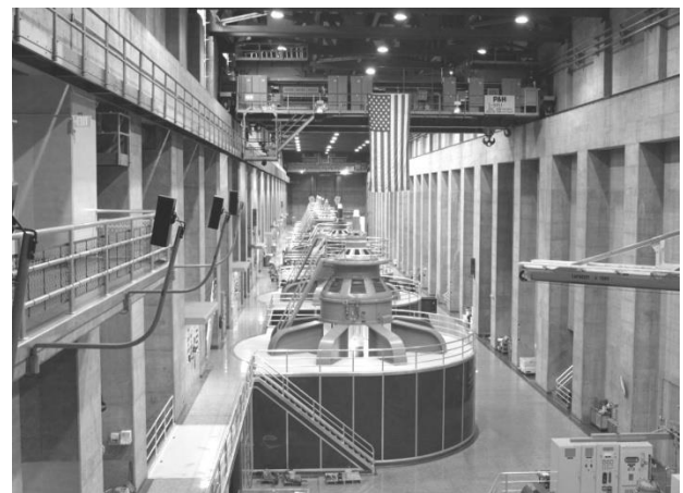
Fig.4 Main Turbine Hall
